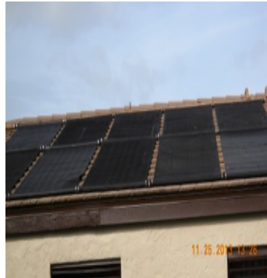
SOLAR POOL HEATING PANELS
